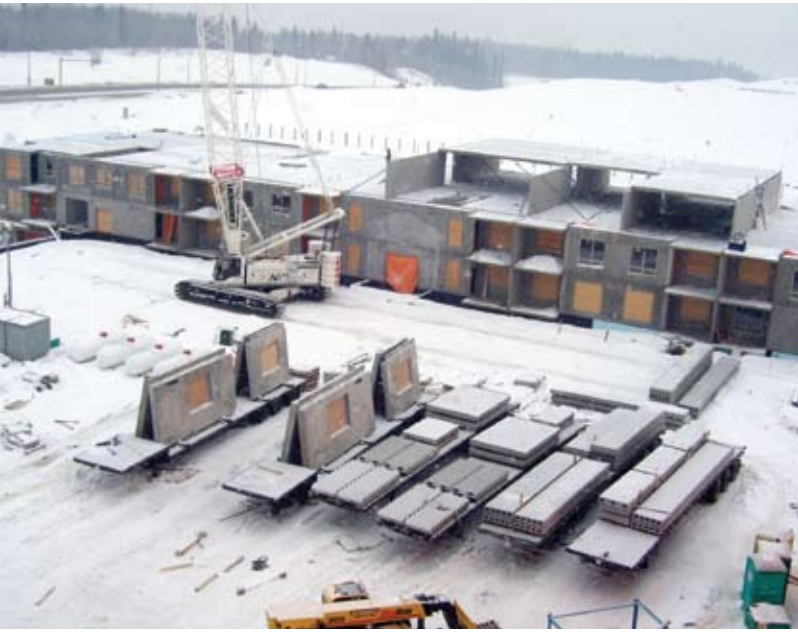
Above The average low temperature in winter at the site of the Eagle Ridge condominiums in Fort McMurray, AB, Canada, is -23^{\circ}\text{C} ( -10^{\circ}\text{F} ). Courtesy of Lafarge.
