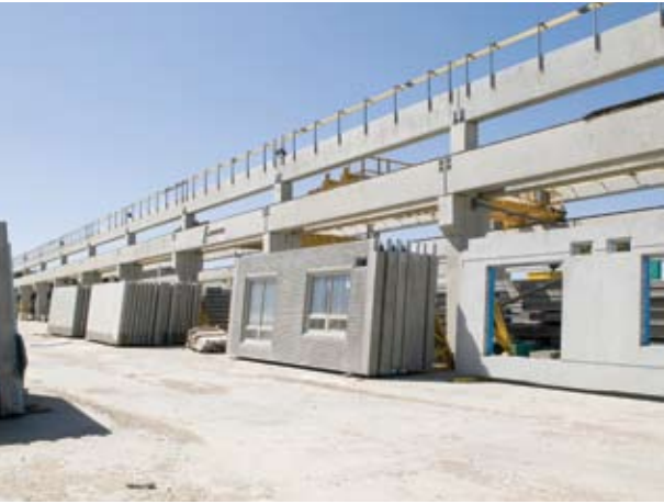
The window contractor installed the windows in the panels at the Edmonton, AB, Canada, plant prior to shipping the panels to the construction site for the Eagle Ridge condominiums in Fort McMurray, AB.
