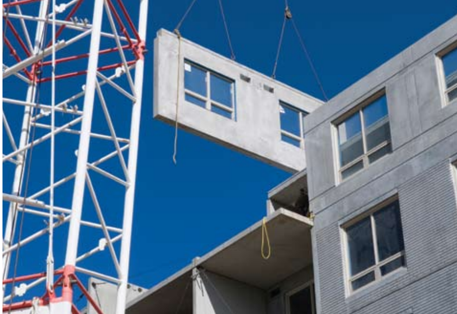
The buildings of the Eagle Ridge condominiums in Fort McMurray, AB, Canada, are assembled like a jigsaw puzzle and can be completed in 62 days. Courtesy of Tucker Photography.
